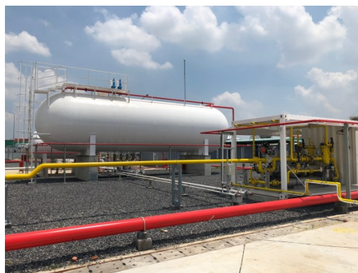
External appearance of the gas supply facility at the Phu My 3 Specialized Industrial Park.
